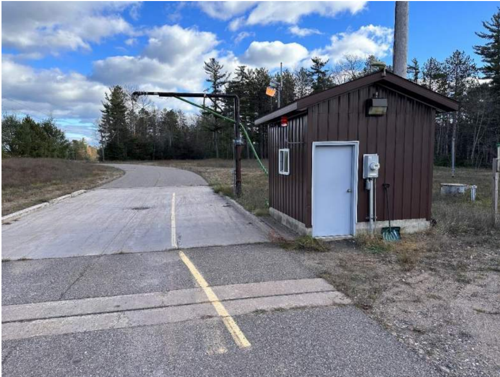
Photo No. 5 – Landfill No. 3 leachate loadout facility.
