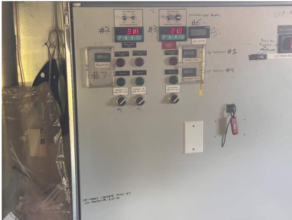
Photo No. 1 – Leachate sump master board readings.
