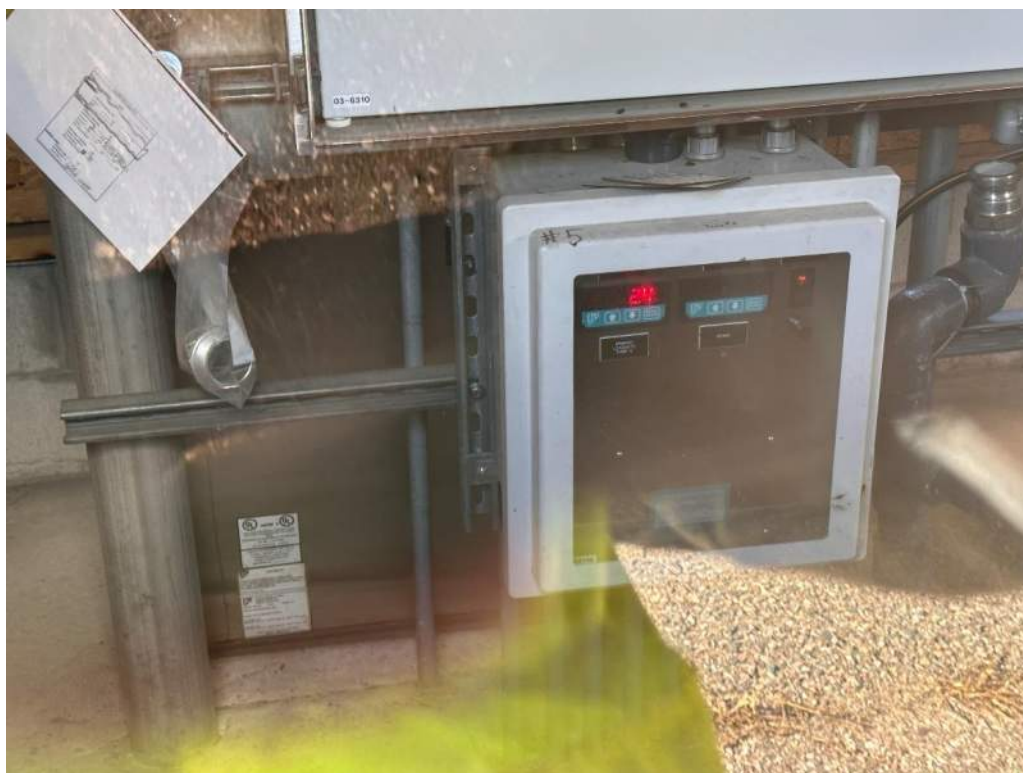
Photo No. 2 – Primary Leachate pump #1-2.
