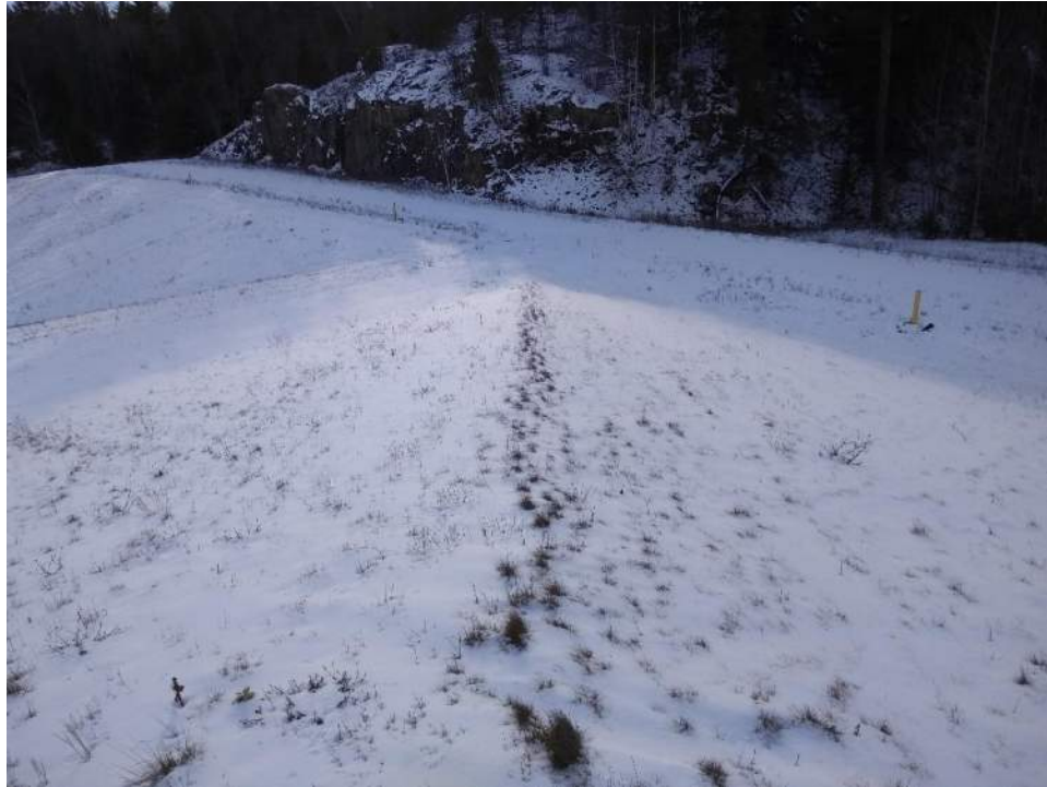
Photo No. 5: Corner of the west and south slope at the PIPP Landfill No. 3, looking southwest.
