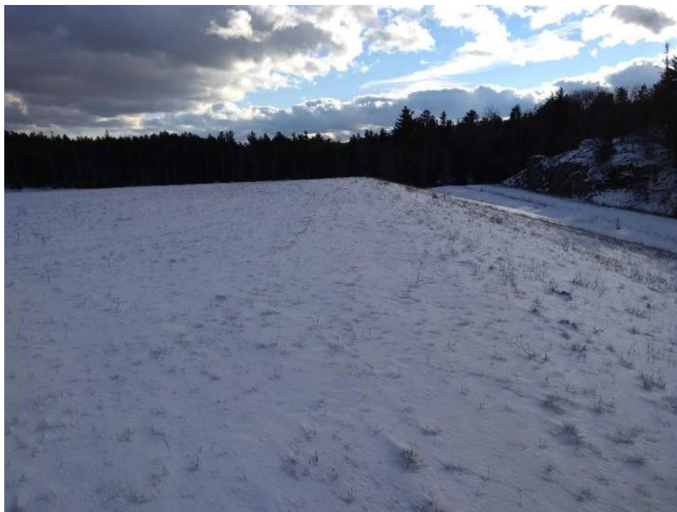
Photo No. 4: Crest of the west slope at the PIPP Landfill No. 3, looking south.
