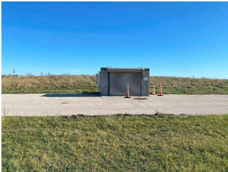
Photo No. 2 – Leachate sump collection vault.
