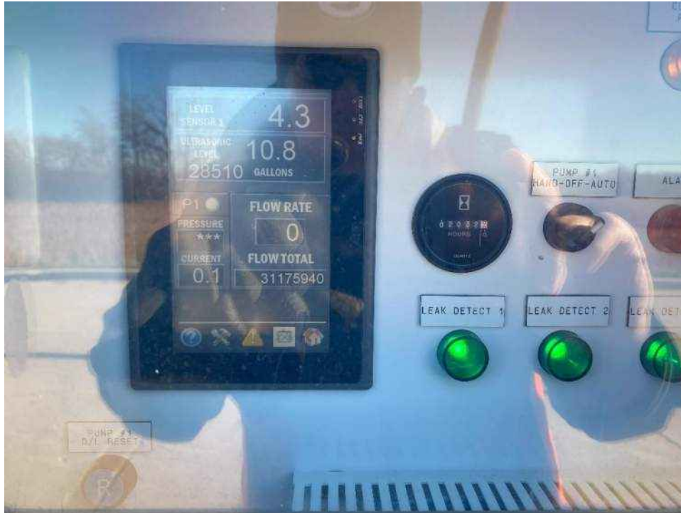
Photo No. 1 – Leachate loadout screen.
