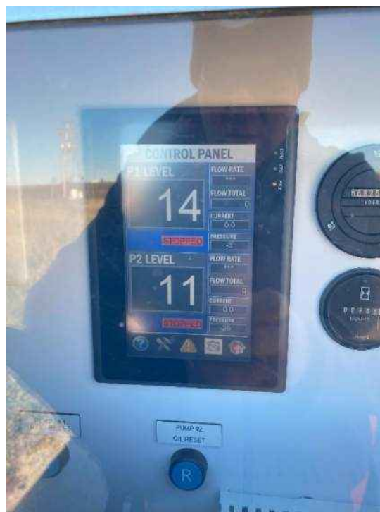
Photo No. 10 – Leachate loadout screen.
