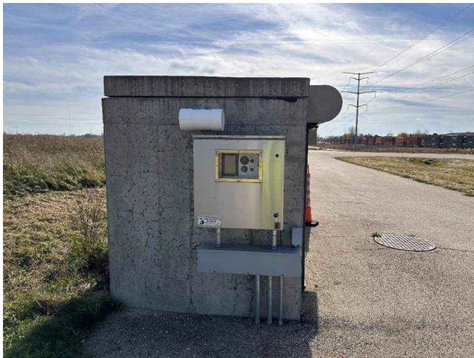
Photo No. 2 – Leachate sump collection vault.
