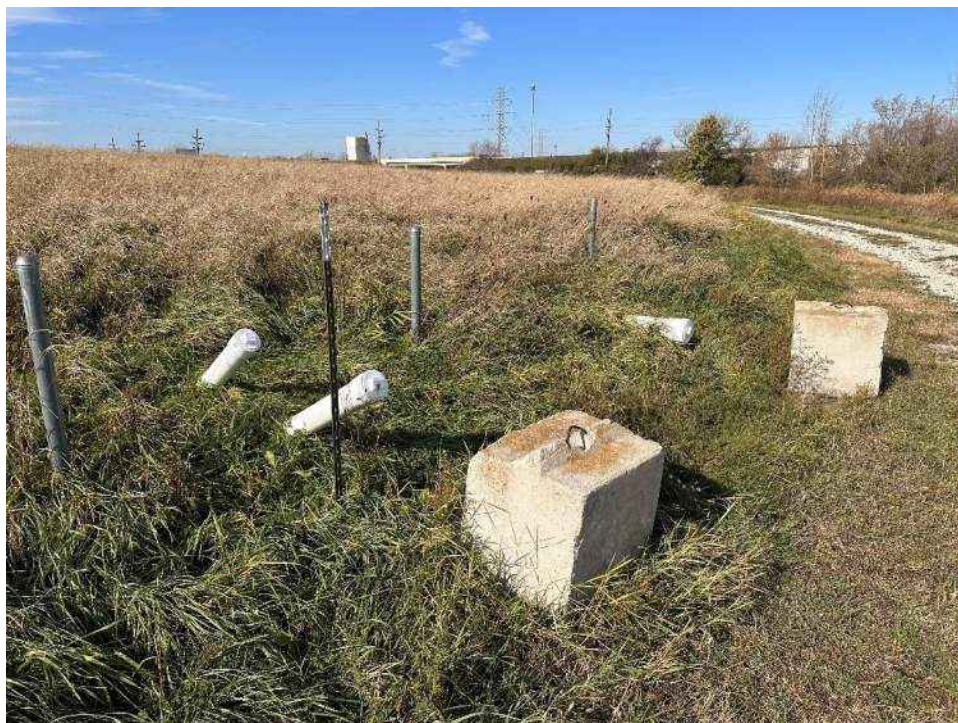
Photo No. 6 – Cleanout and leachate headwell on the east end of Cell 1.
