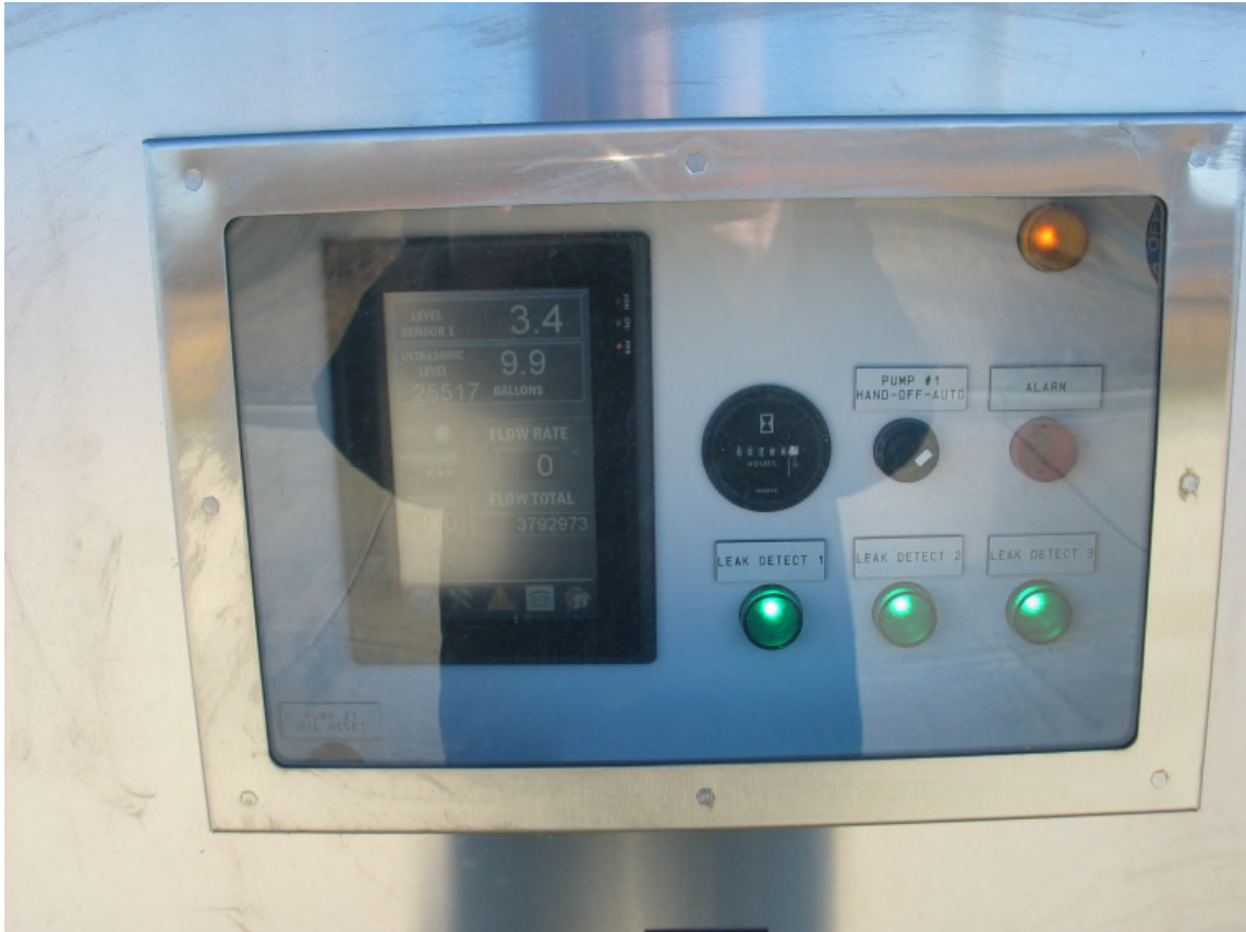
Leachate Storage & Load-Out Control Panel
