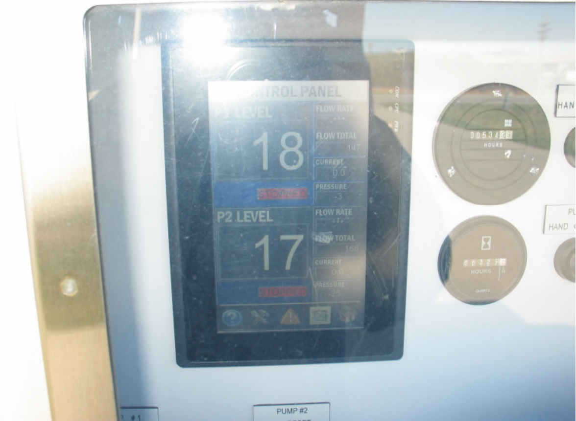
Sump Transducer Readings/Control Panel
