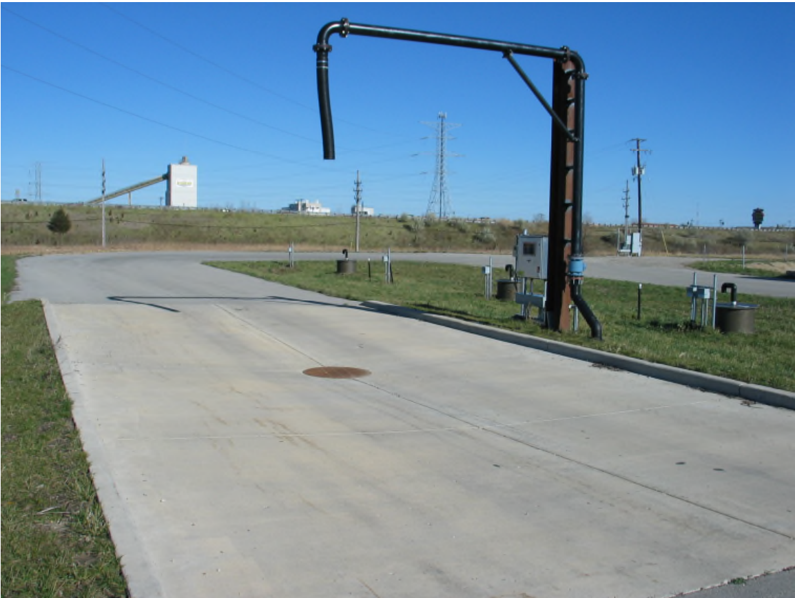
Leachate Load-Out (looking north)
