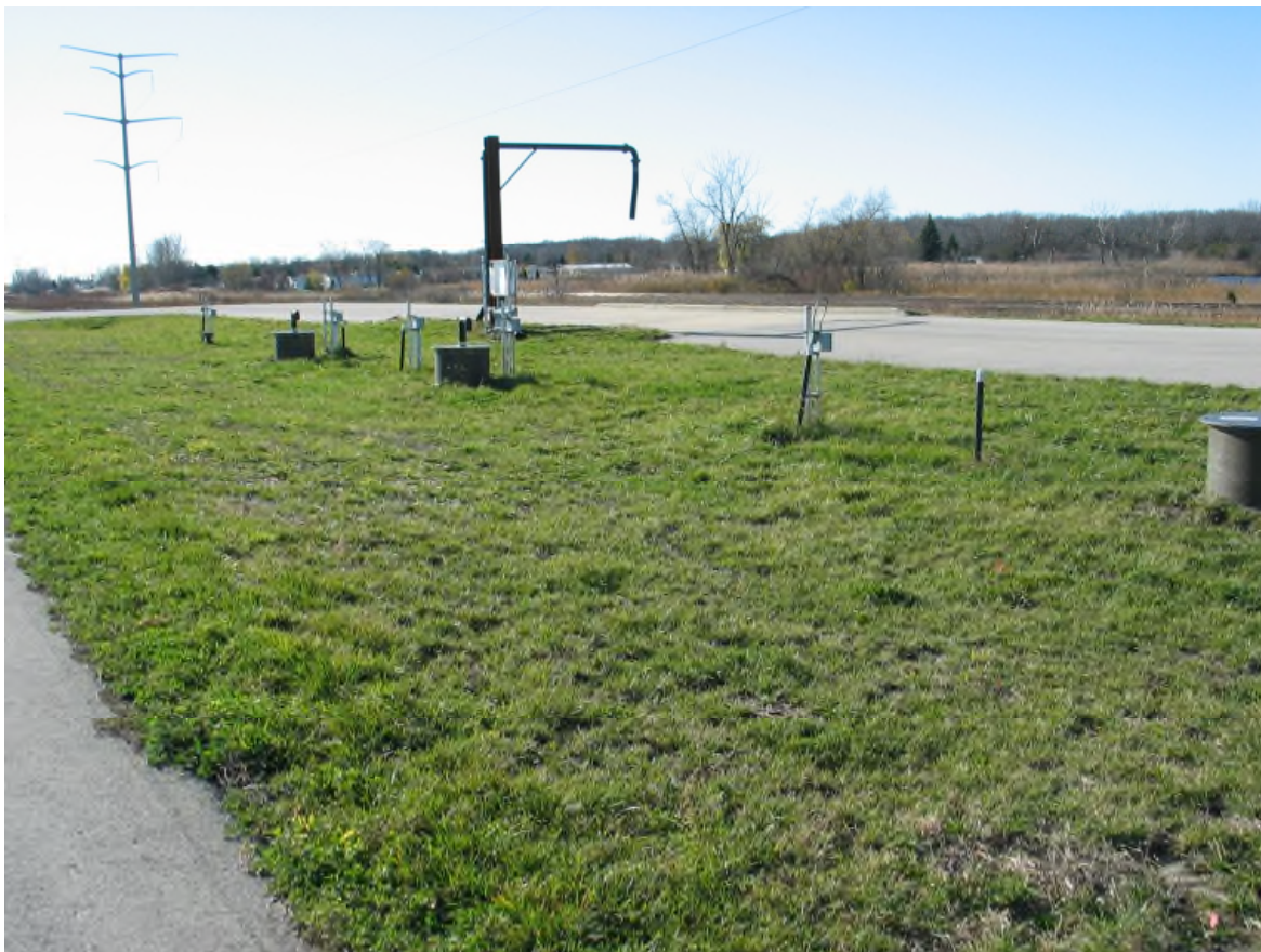
Leachate Storage Tank and Load-Out (looking southwest)
