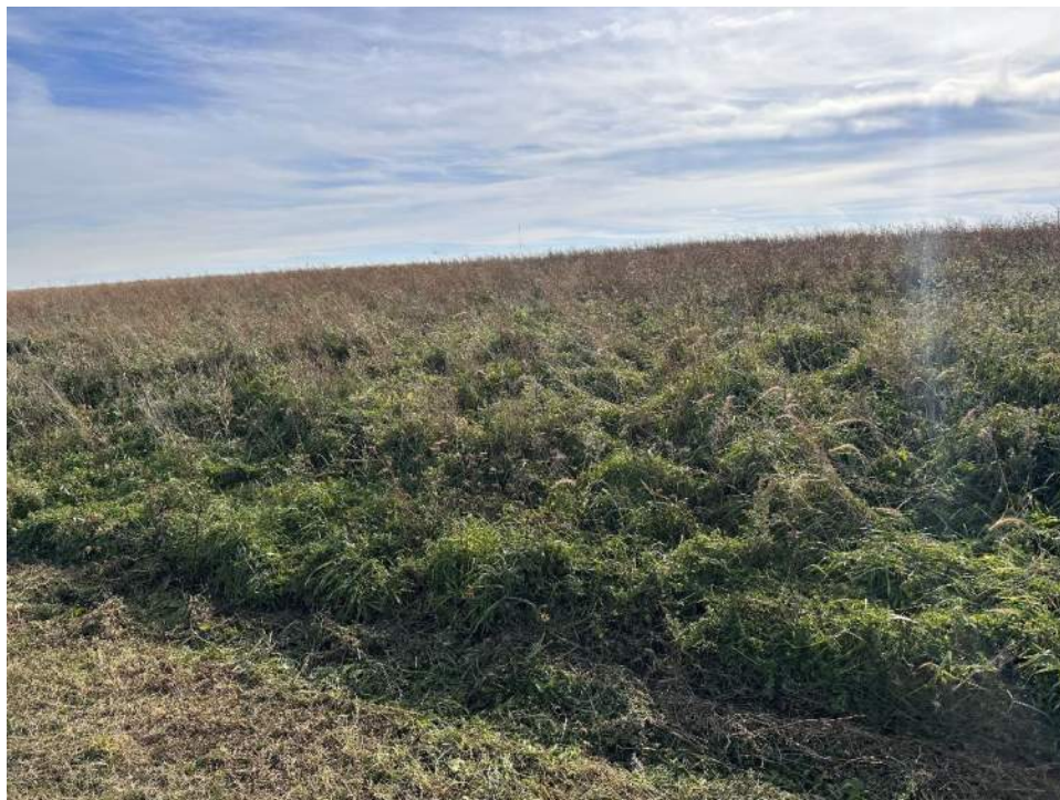
Photo No. 4 – North slope of Cell 1, looking southeast, showing thick vegetation.
