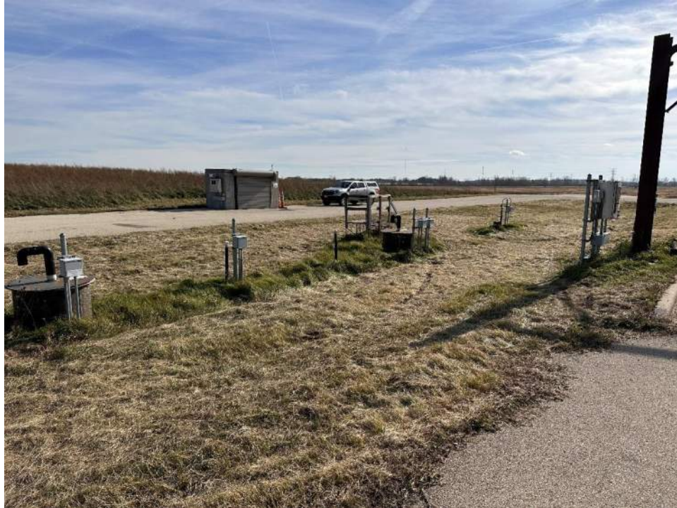
Photo No. 1 – Looking southeast at underground leachate storage tanks.
