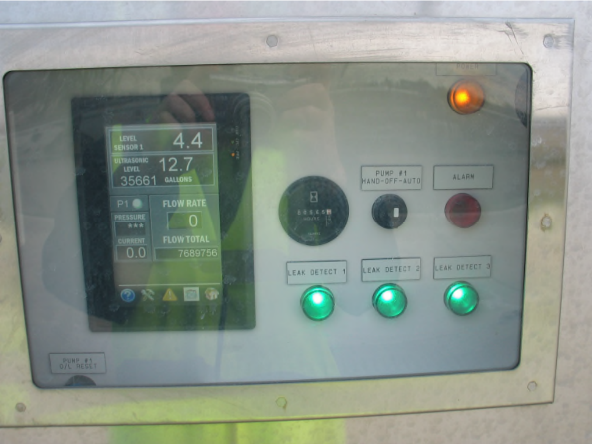
Leachate Load-Out Panel
