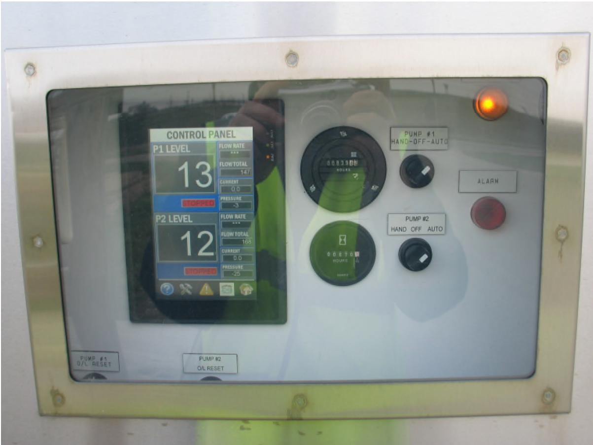
Sump Transducer Readings/Control Panel
