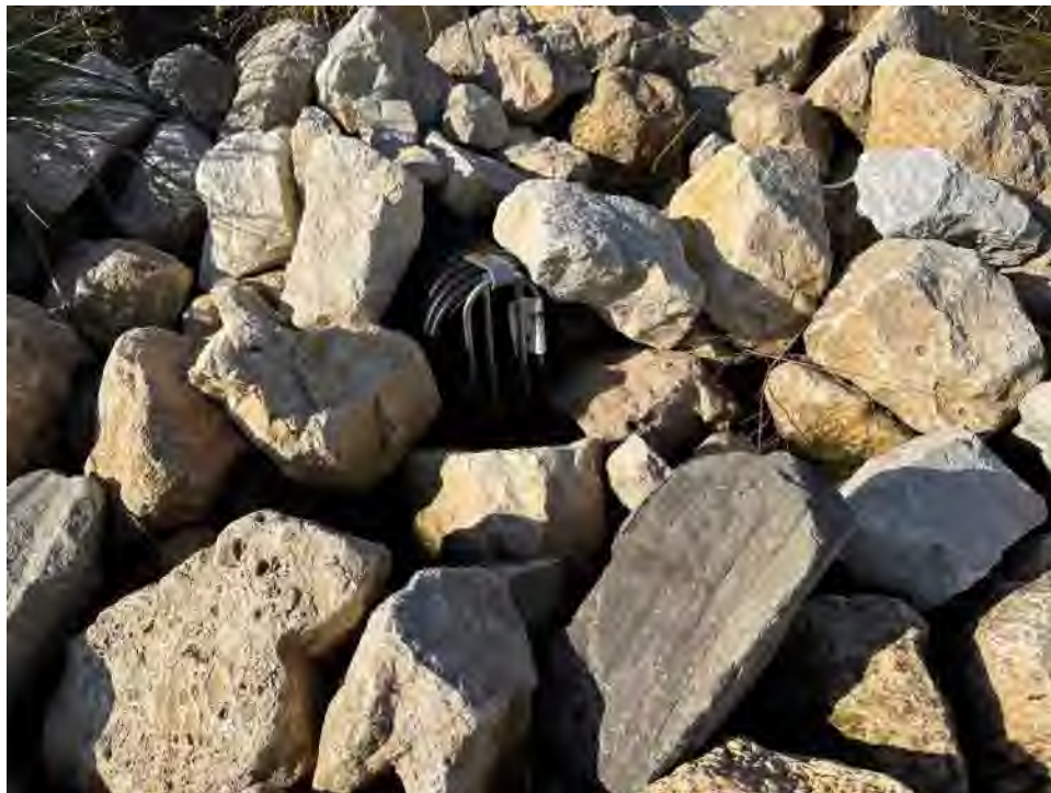
Photo No. 8 – Cover drain outlet at the toe of the Cell 6 and 8 slope.
