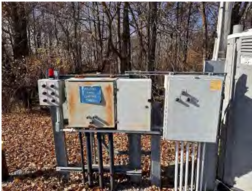
Photo No. 10 – Leachate tank control panel.
