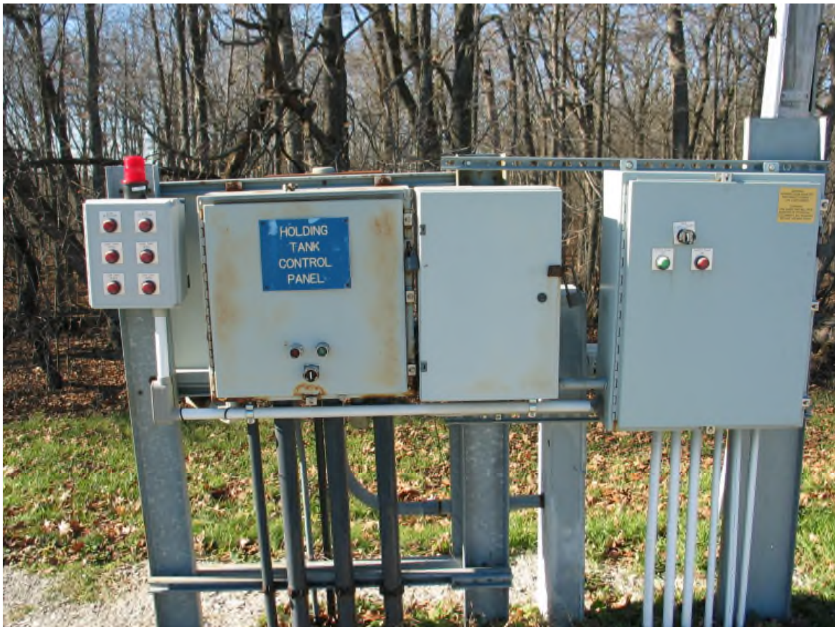
Leachate Load-Out & Storage Panel
