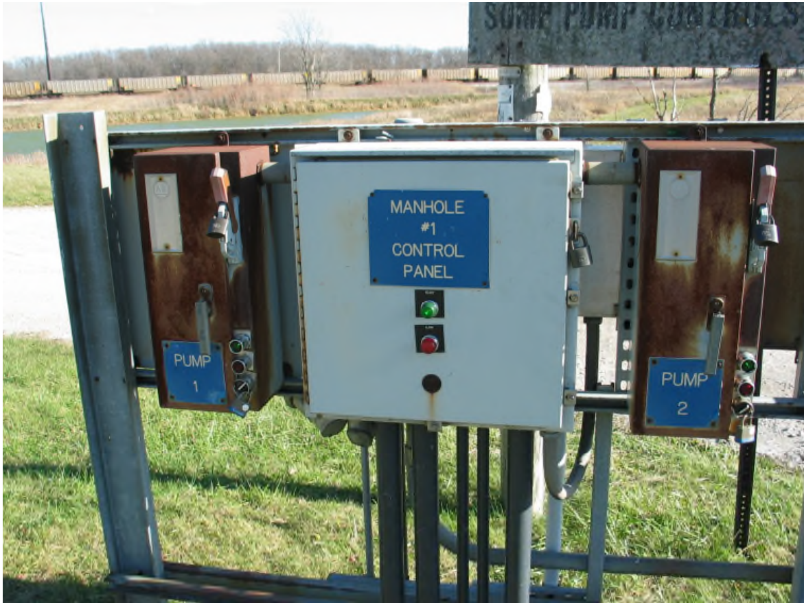
Lift Station Controls
