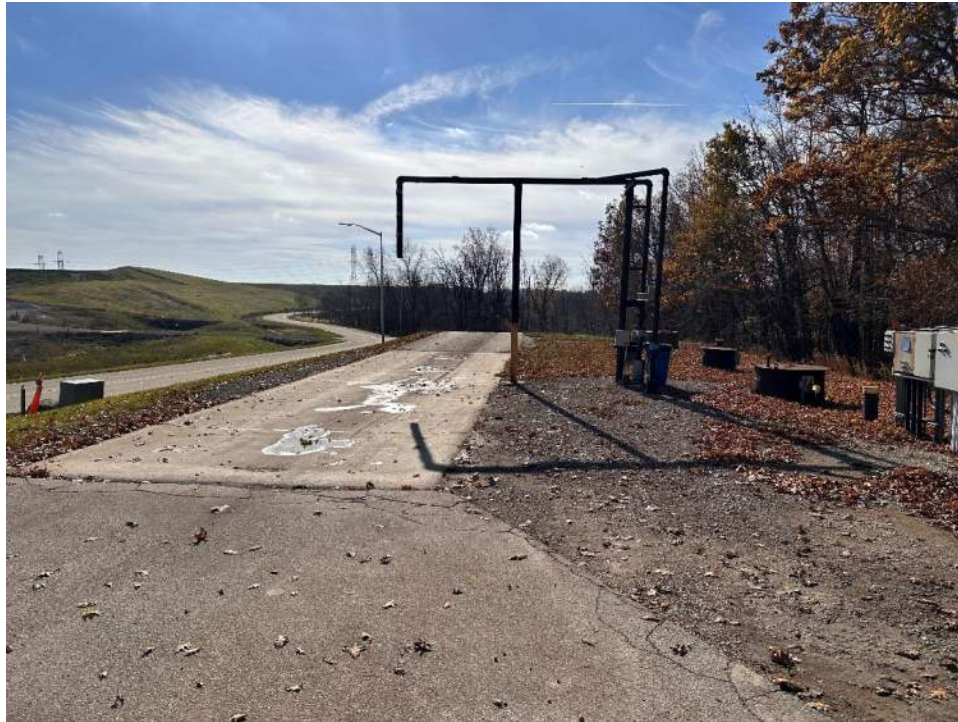
Photo No. 9 – Leachate load-out facility.
