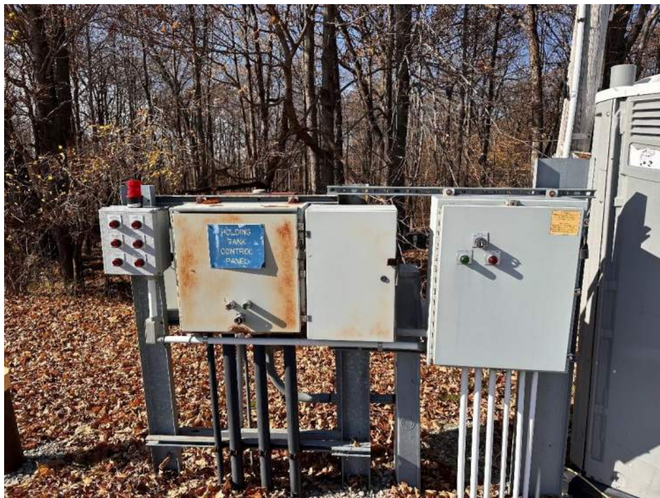
Photo No. 10 – Leachate tank control panel.
