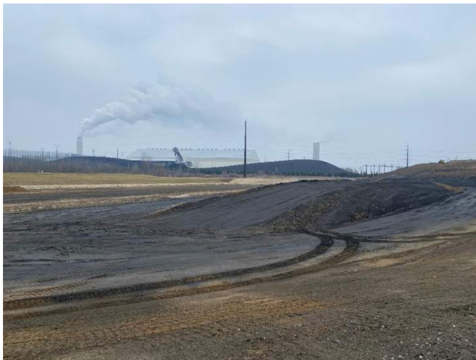
Photo No. 2: Bottom ash stockpiled for beneficial use inside Cell 10 looking west on 12/07/2022
