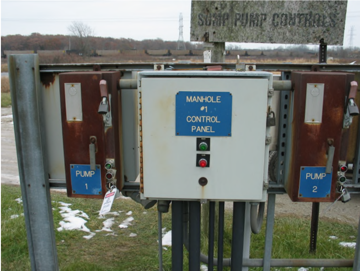
Lift station controls
