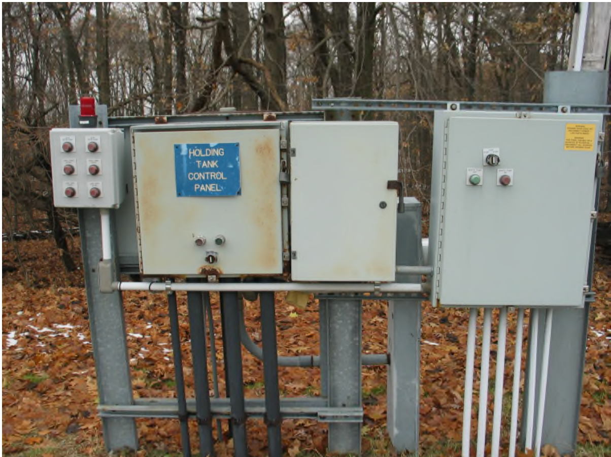
Leachate load-out controls
