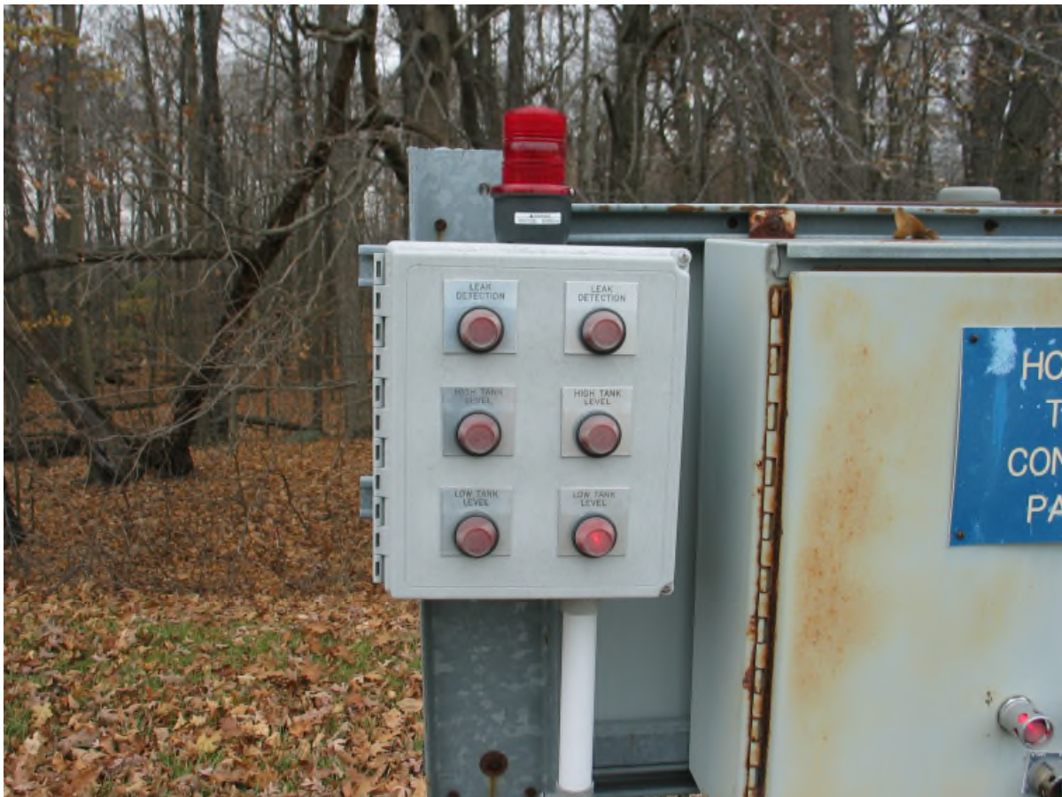
Leachate Load-Out Alarm Panel
