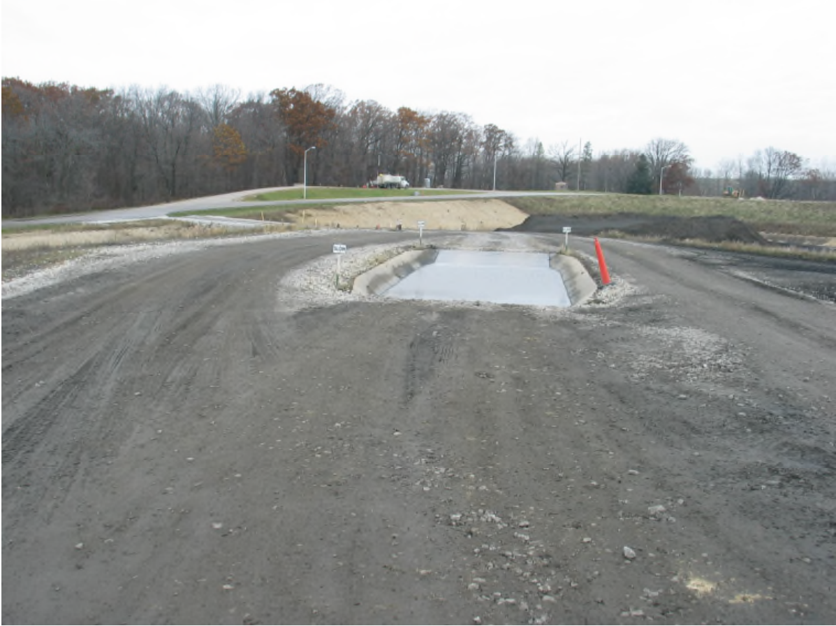
Tire Wash (looking north)
