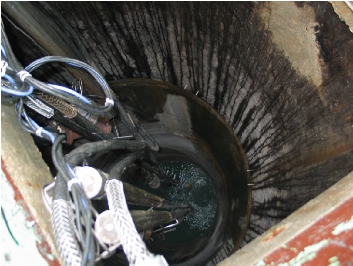
Lift Station (looking down)
