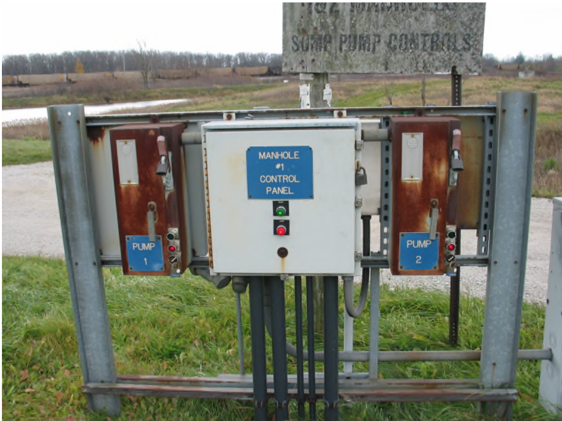
Lift Station Control Panel
