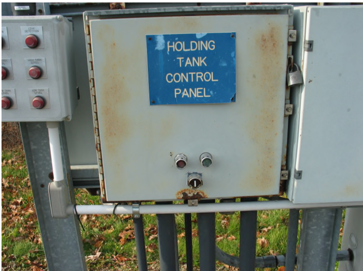
Leachate Load-Out & Storage Panel
