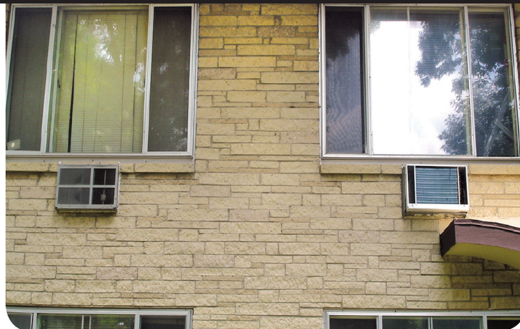
Old low efficiency unit (left) side by side with new high efficiency unit (right)
