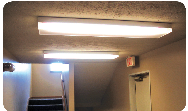
New high efficiency T8 fluorescent and LED exit fixtures
